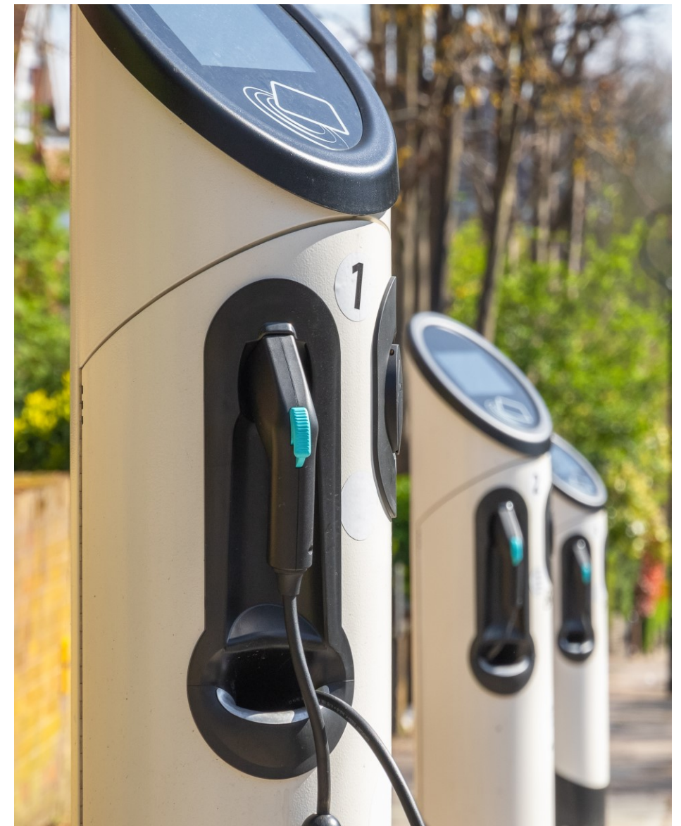
Figure 3 EV Charging Point
